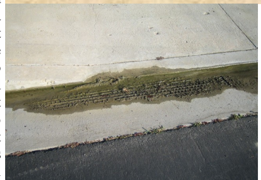
Mud and Debris in HOA Gutters.
