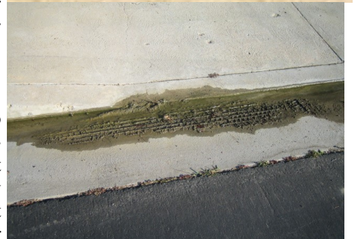
Mud and Debris in HOA Gutters.
