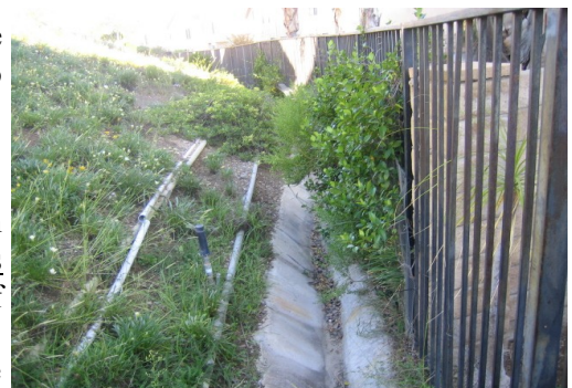
Overgrown Material on Common Area
